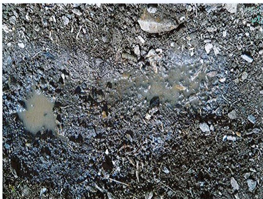
Fig 2.4: photo showing evidence of water logging
